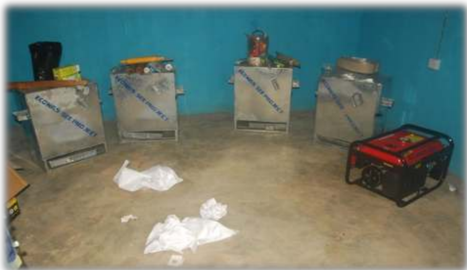
Figure 4: Ovens and some other catering equipment and power generator
